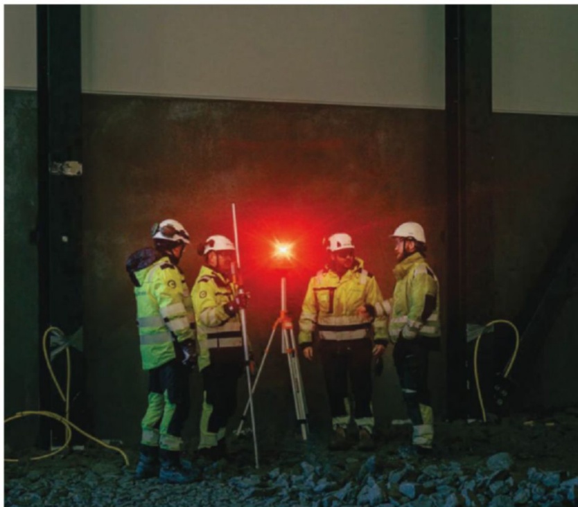
▲ Workers inside an in-progress data hall at Nscale’s Narvik data- center site on March 20
