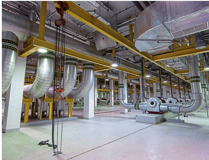
Some district cooling networks already exist in places like Dubai
